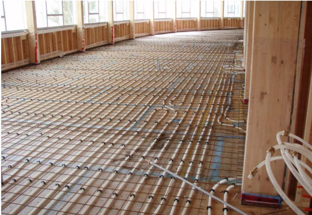
Figure 3.2: Second floor of the Living with Lakes Building. The in-floor radiant heating tubing is installed and ready for the concrete to be poured over. Source: VLWLC 2012
