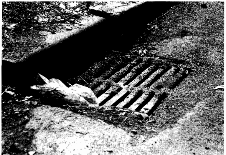
FIGURE 20.7. Stormwater drainage. (Photo by J.M. Gunn.)
